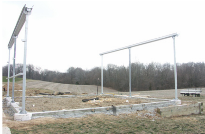
Fig. 1: New research greenhouse under construction at the Southwest Purdue Ag Center. (Photo by Dan Egel)
