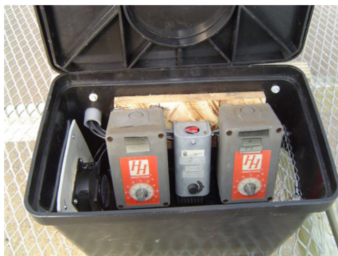
Figure 1. Example of thermostats in a box with a fan. Box will be painted white.
